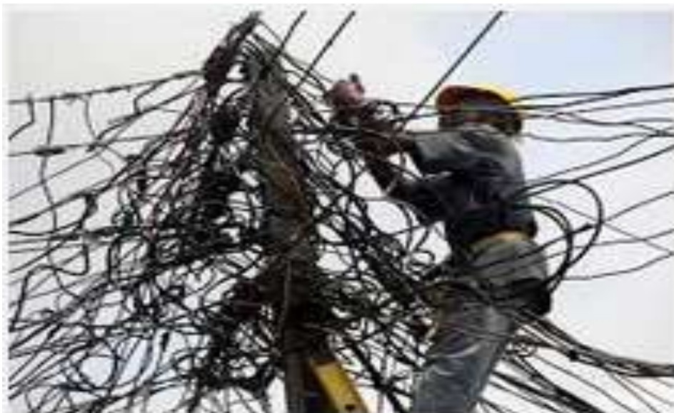
Fig. 2 Typical Maintenance Handling At Nigeria's Distribution Networks
