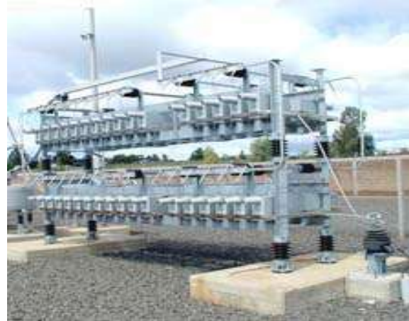
Fig. 9 Block of commercial used capacitors
