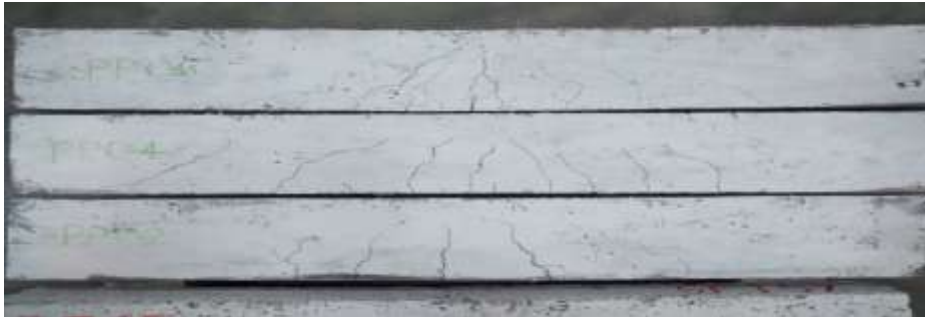
Figure 7: Cracked Polypropylene Fiber Reinforced Beam
