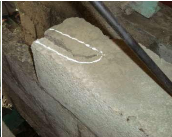
Fig.8 Crack in hollow concrete block wall.
