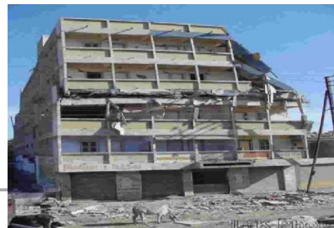
Fig. 2 Floating Column building failure
